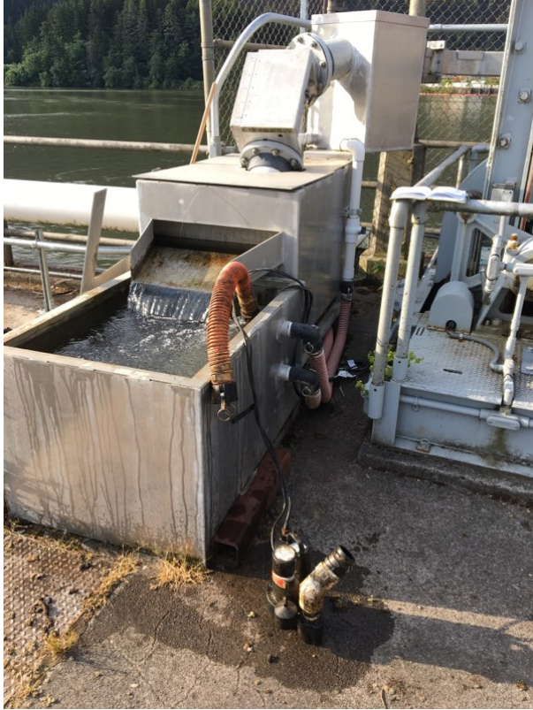
Figure 2. Two pump set up used to lift water from the new forebay extension to the older climbing section. Failed pump removed.
