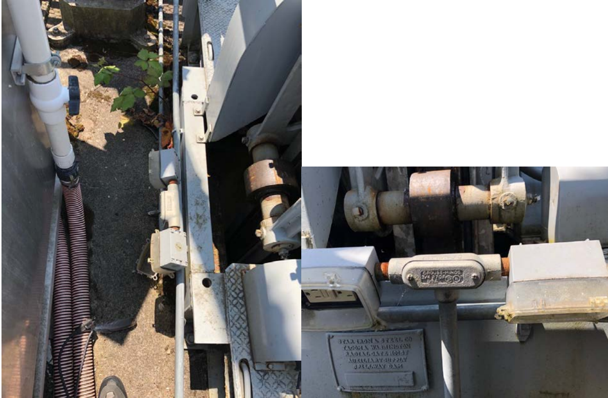
Figure 3. Two GFI outlets that power the 110 volt a/c pumps. Both were found tripped on the morning of 4 June so no water was flowing through the climbing section. The right one would reset and pump would operate, the left one would trip each time the failed pump was plugged in.
